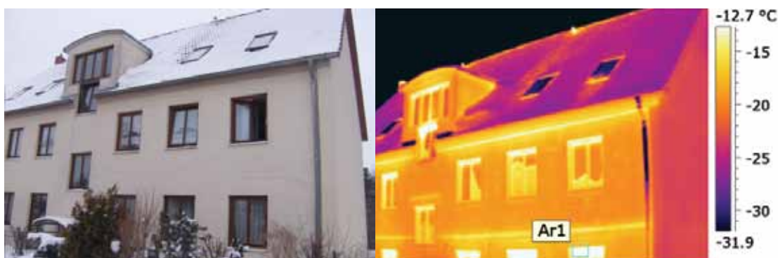
In this example it is clear that the rightmost skylight is leaking warmth at the frame and there are several locations where the roof insulation isn't very effective.
